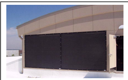
Louver Intake Filters
