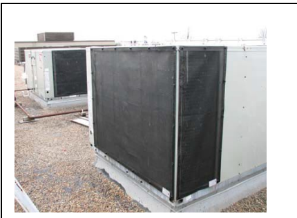
Rooftop Unit Filters
