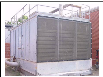
Cooling Tower Filters
