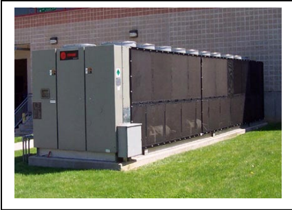
Chiller Coil Filters
