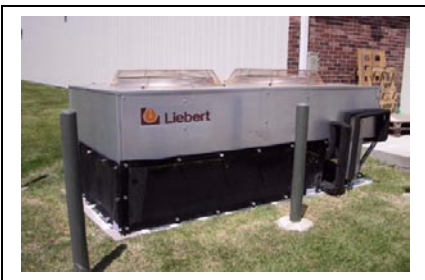
Dry Cooler Filters
